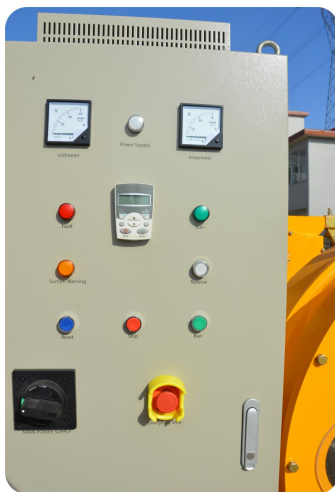
Nice quality electric control box
